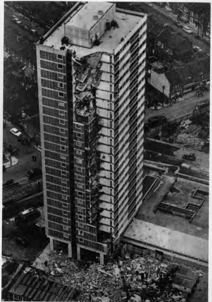
Ronan Point, London, UK, Taylor Woodrow-Anglian, 1968. This progressive collapse caused by a gas explosion signalled the end of the precast-concrete era.
