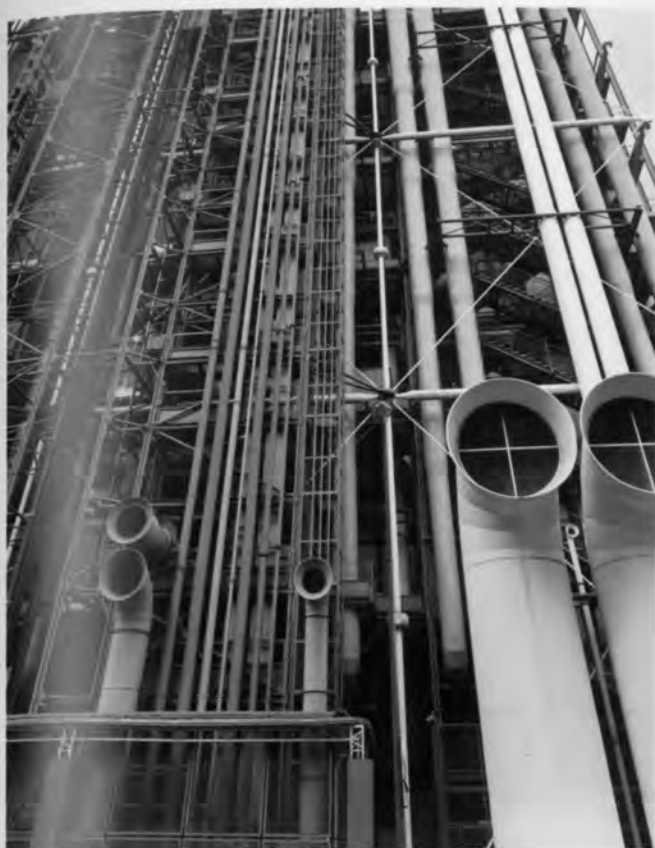
(Above) Centre Pompidou detail. Exposed pipes and ducts on the Rue du Renard side of the building.
